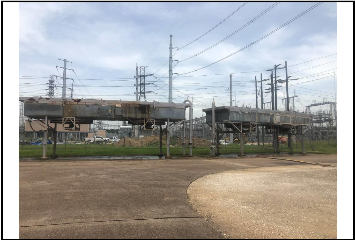
Photo 7: Gas Turbines 83-84 Cooling Skid, facing east.
