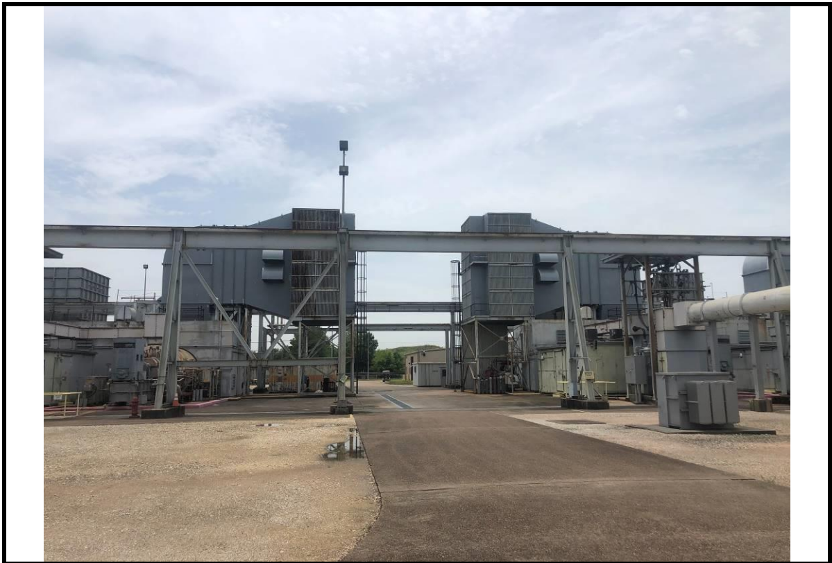
Photo 6: Gas Turbines 81-82, facing west.
