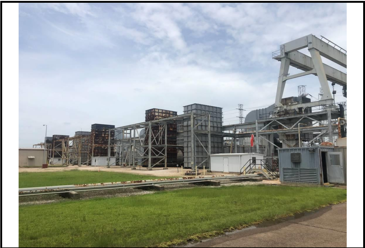
Photo 4: Gas Turbines 70s and 80s, facing northeast.
