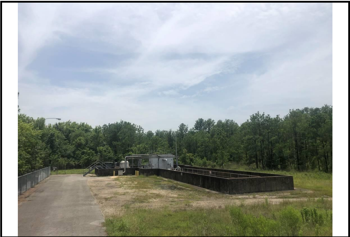
Photo 10: Tricellerator, facing southwest.
