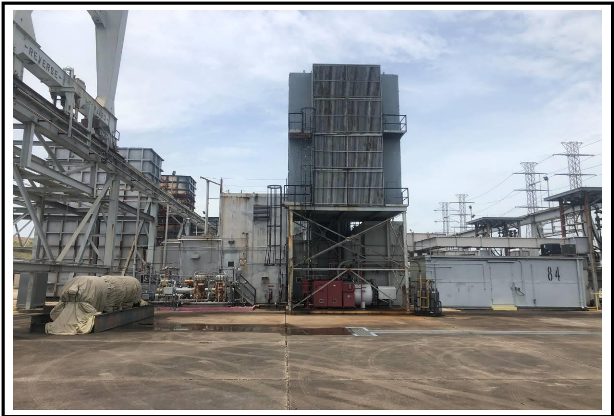
Photo 8: Gas Turbine 84, facing north.
