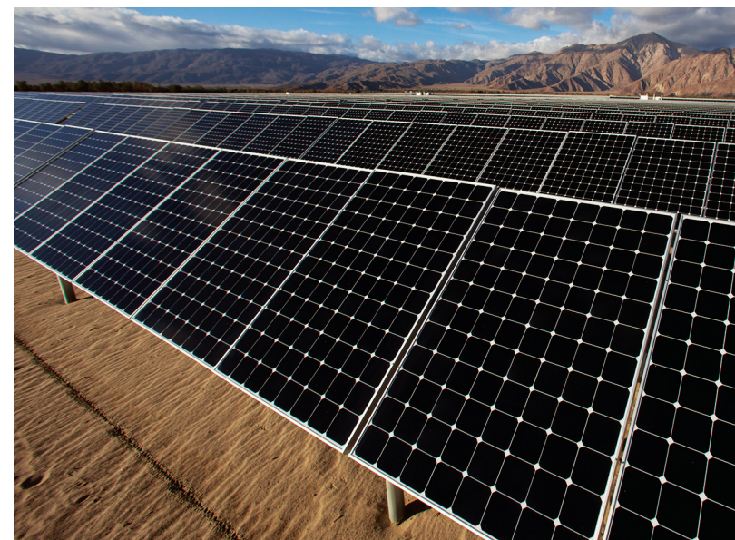
Borrego Solar Generating Station, CA
