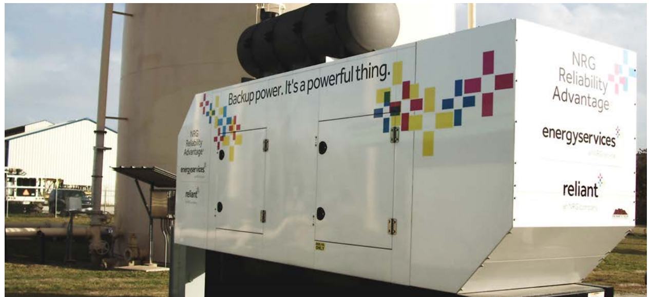
An NRG Reliability Solutions backup generator
